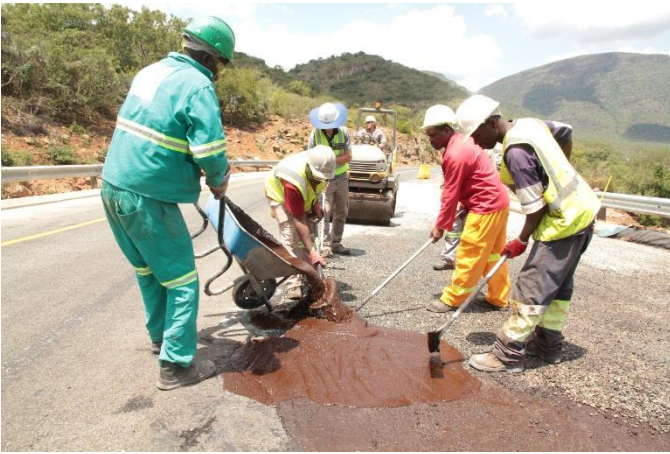
Fig.6 Final placement of the composite Macadam layer, showing the combination of labour and two ton sit-on roller.
